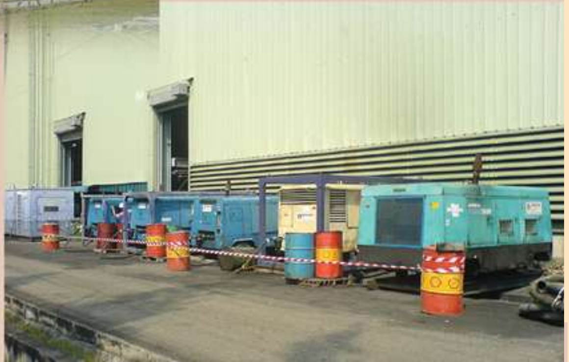
Kapar Power Plant
